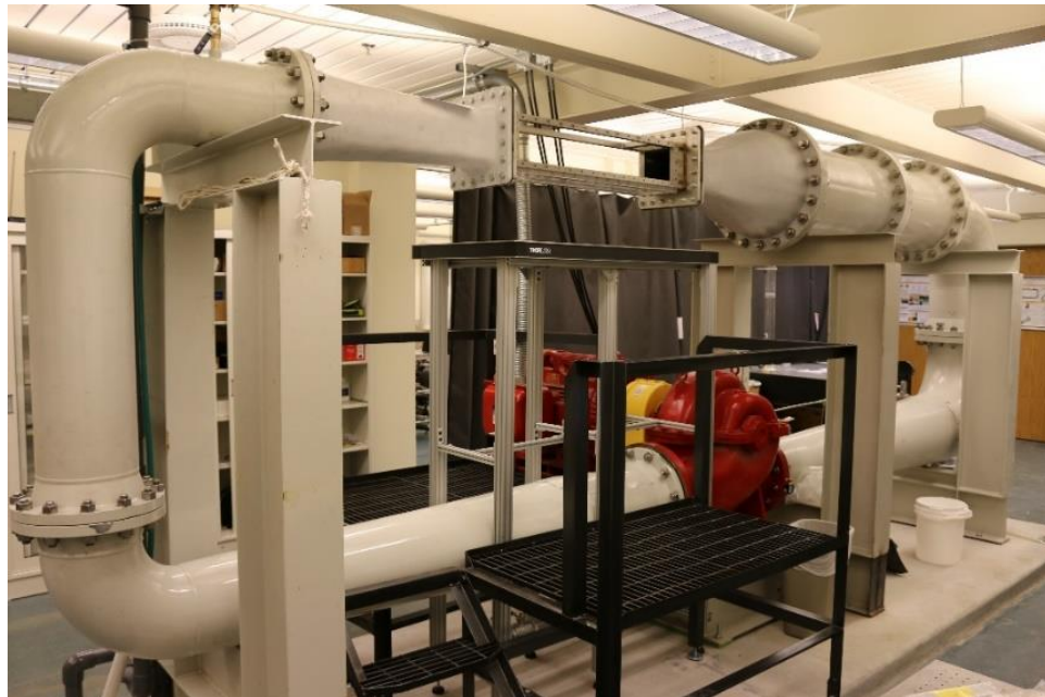
Figure 3-2. Picture of the installed water tunnel with the pump/motor on the lower leg (in red) and the test section almost directly above on the pump/motor.
