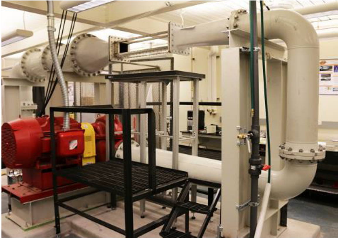
Figure 2.1: EFPL Large Water Tunnel at OSU
